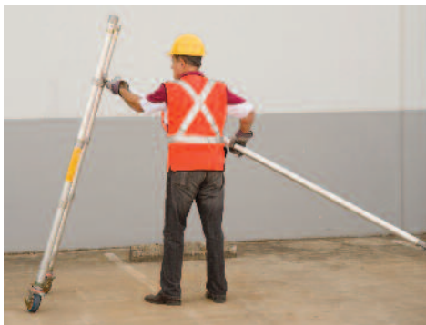
1. Snap short brace (horizontal) onto vertical tube of lower end frame. This supports the frame during installation of the other braces.
